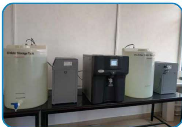
Ultrapure water purification system
